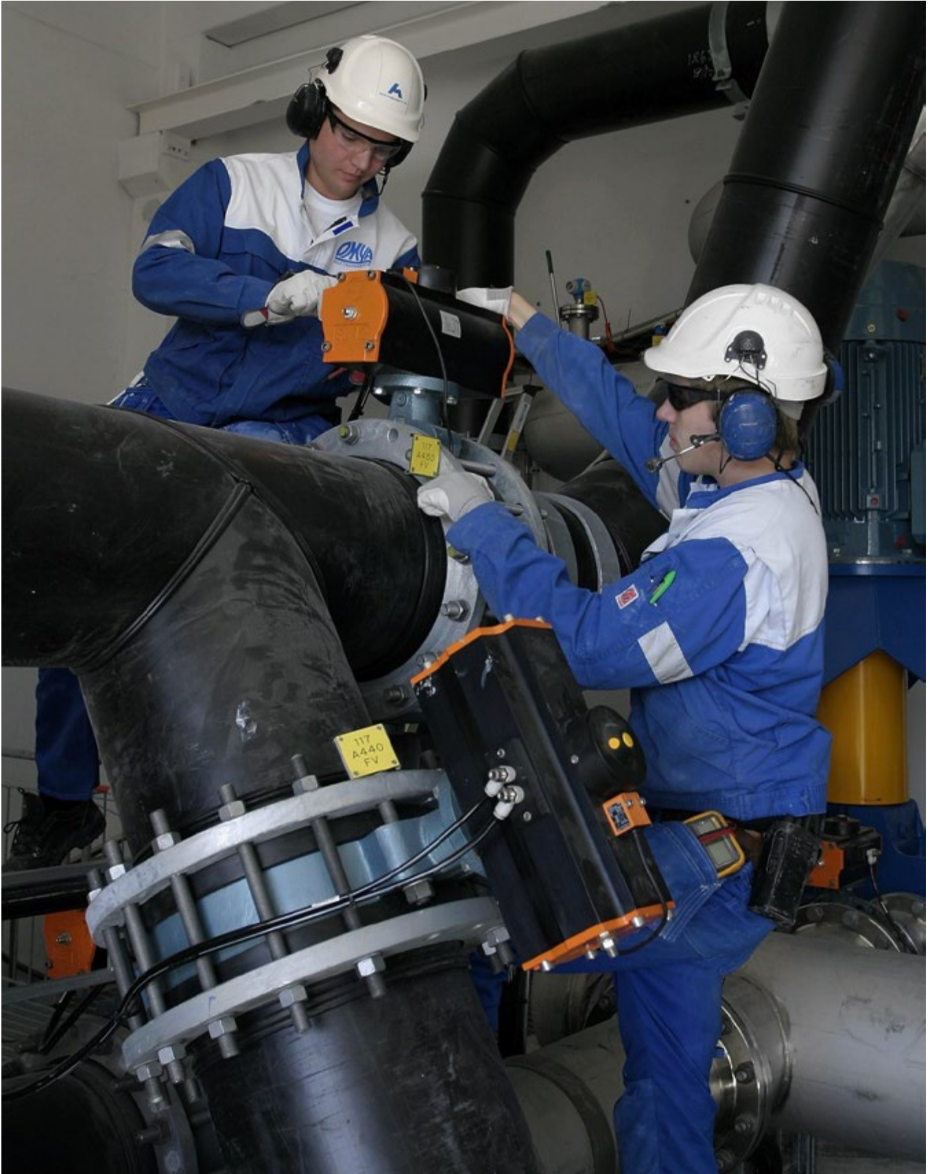
Mounting a control valve in a cooling circuit. The work is being carried out by apprentices at Hustadmarmor AS: Photo: Hustadmarmor A/S
