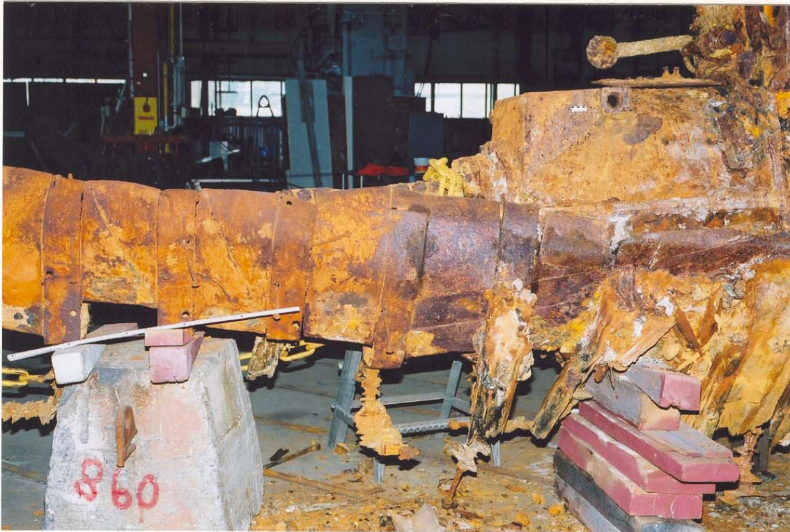
Figure 34 (03/12A): Engine starboard side showing upward bending of foundation plates.
