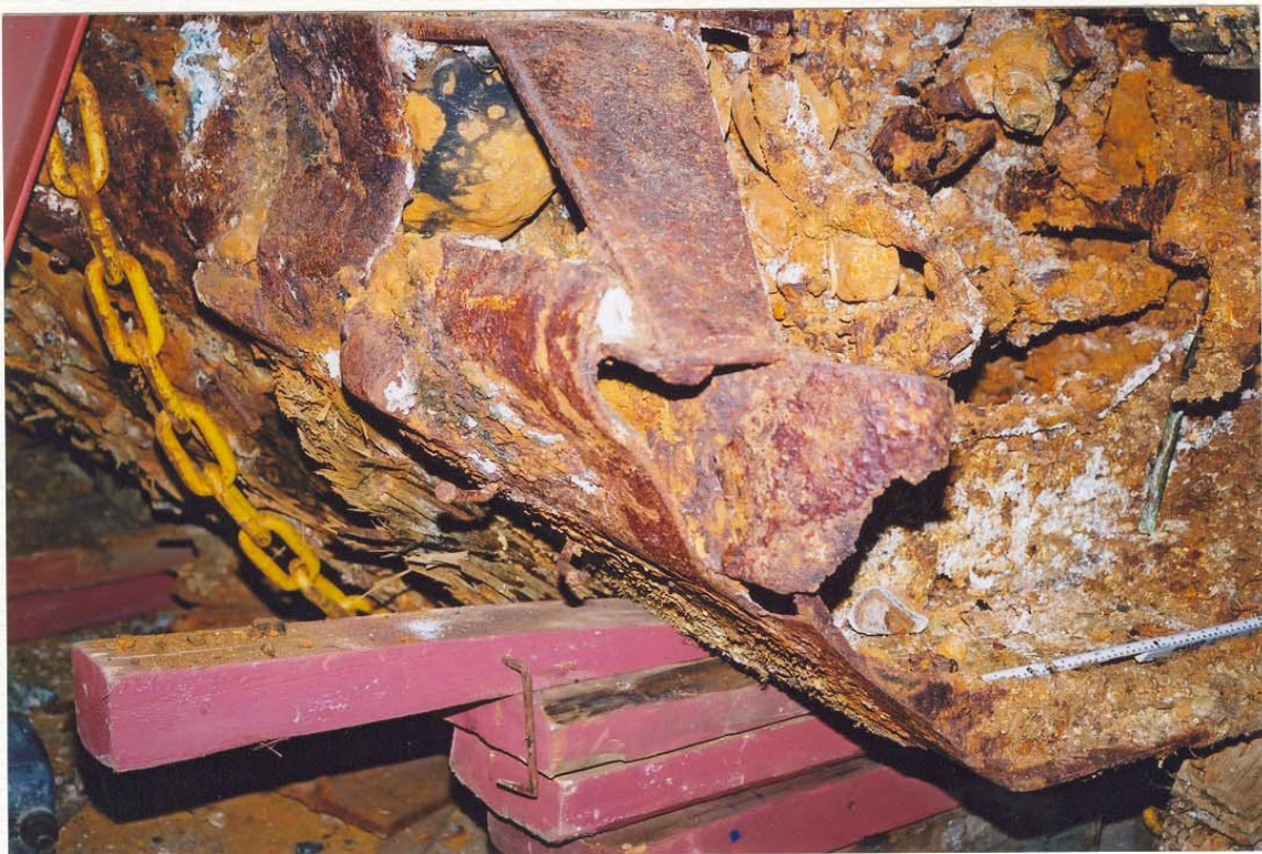
Figure 31 (02/17): Detail of upwardly bent forward starboard side engine foundation plates.
