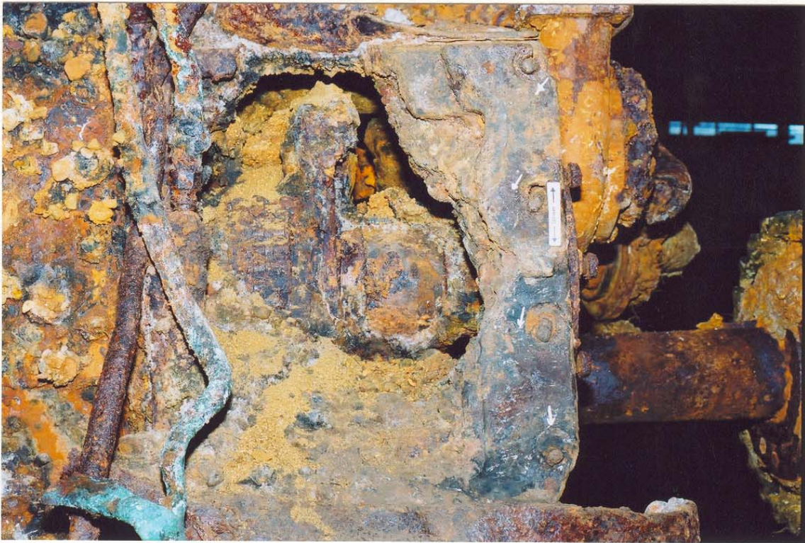
Figure 3 (5/11): Detail of figure 2, showing general direction of stud bending (arrowed).
