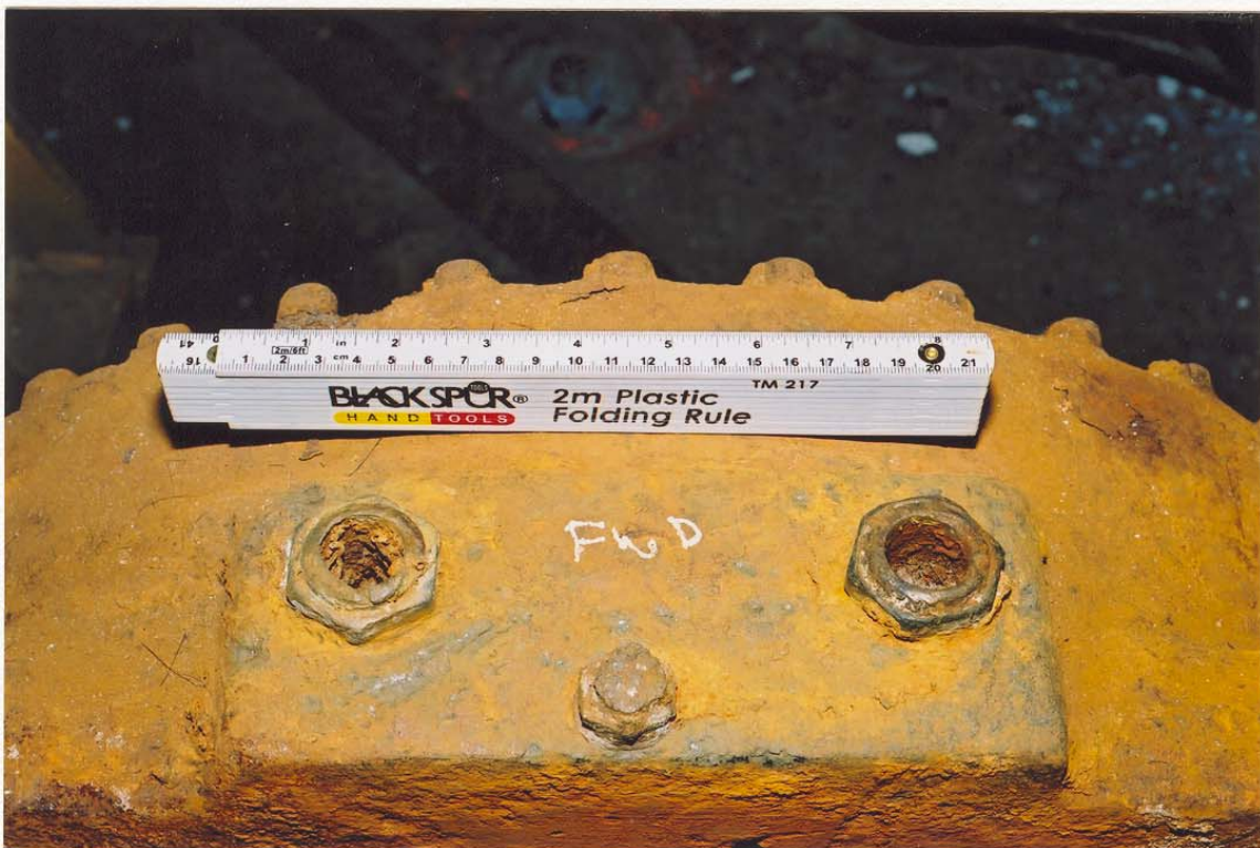
Figure 47 (7/18A): Detail of fractured pilot motor hydraulic pipe connections.
