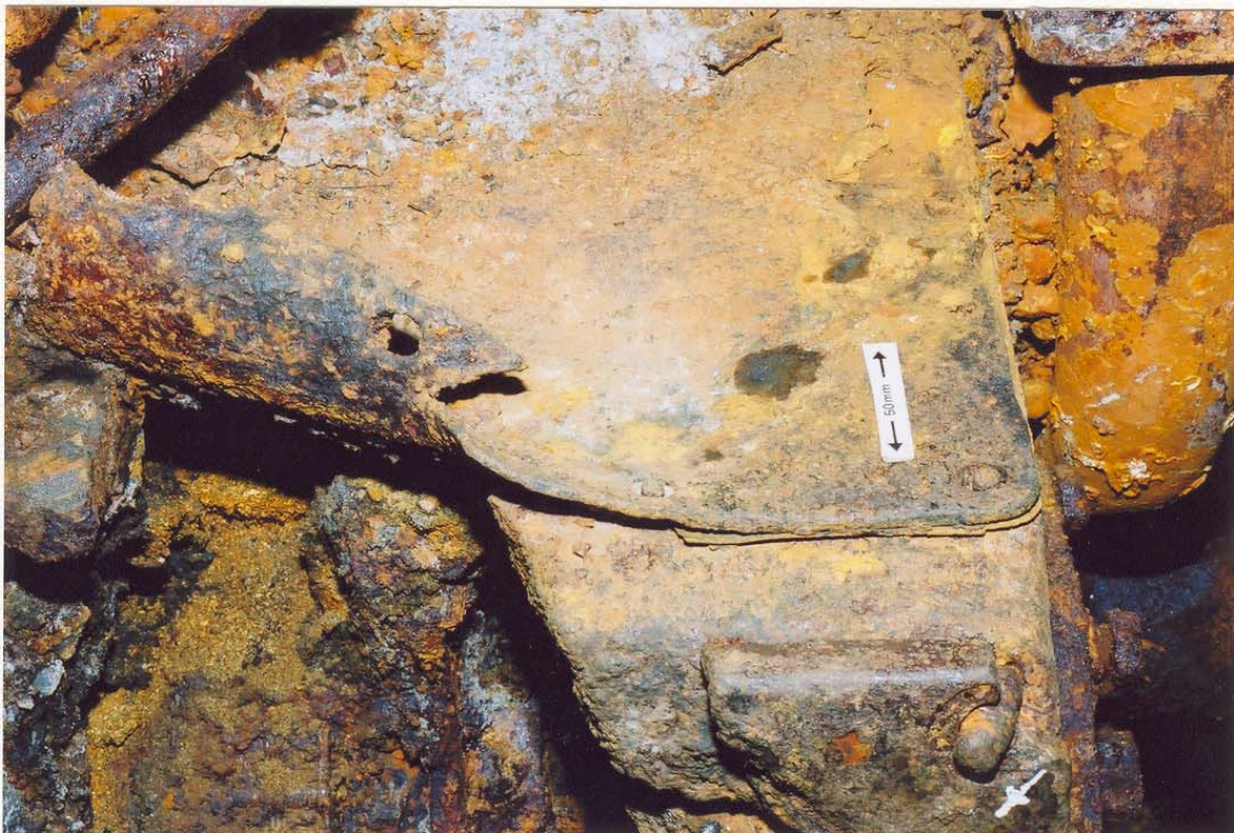
Figure 4 (05/13): Detail of figure 2, showing upward bending of top cover plate.
