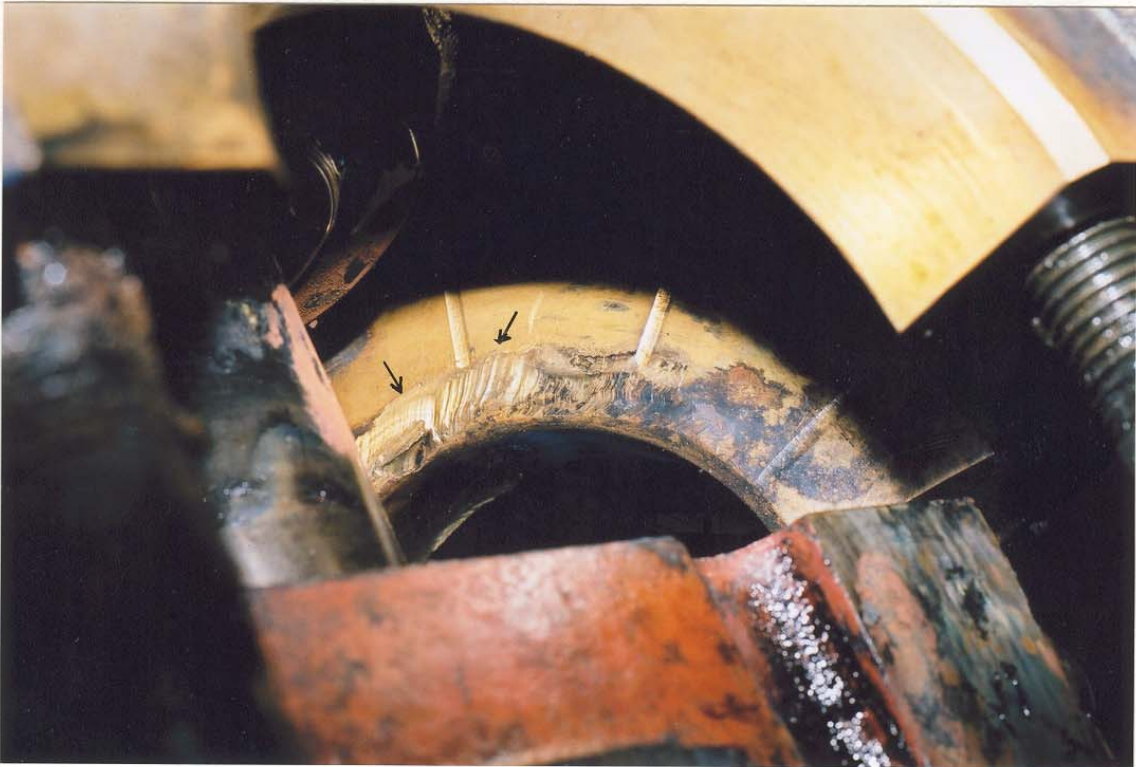
Figure 42 (06/12A): Detail of propeller cone internals, showing severe local mechanical contact damage (arrowed).
