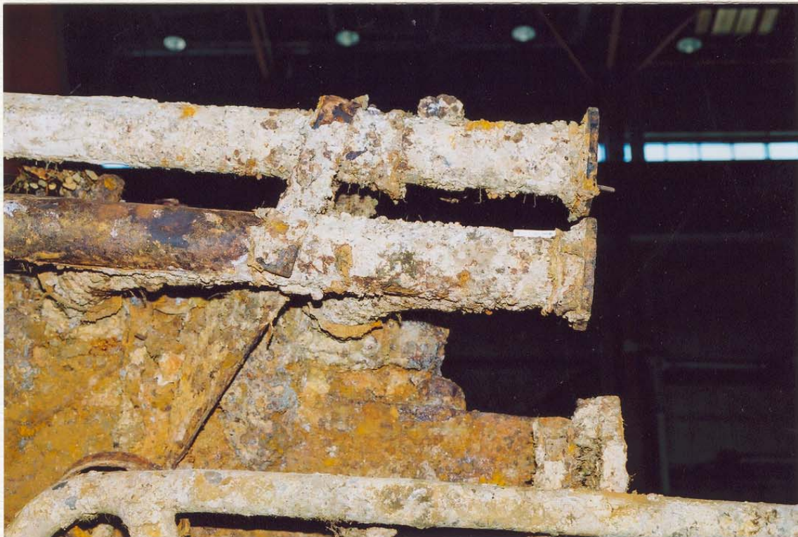
Figure 12 (08/16A): Exhaust flange connections - viewed from aft port side.
