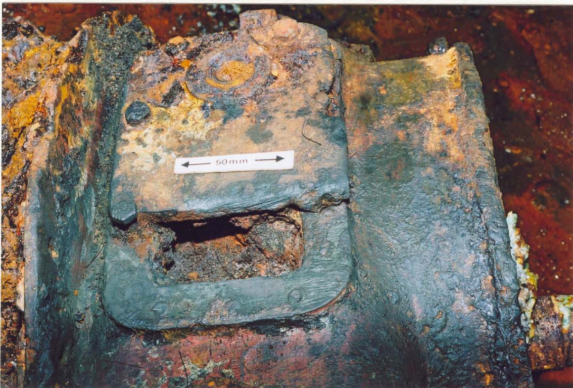
Figure 23 (3/2A): Detail of turbocharger showing fractured cover-plate.
