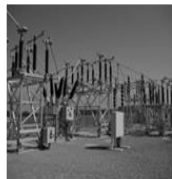
Electrical and power distribution systems
