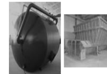
Tanks and mechanical structures
