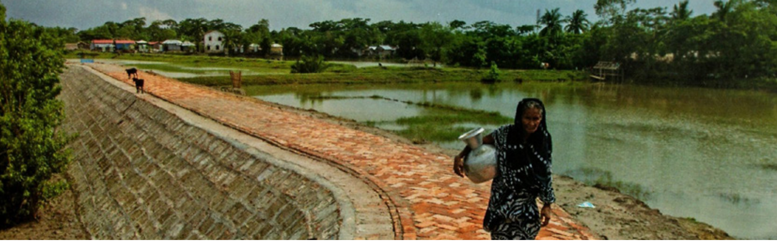
Construction of dikes is one of the measures undertaken to prevent floods from causing major destructions, in a country strongly exposed to natural disasters including floods and cyclones. (Photo: UNDP)
