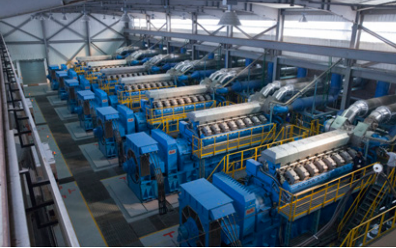
Generators from Bergen Engines (Norway) are producing more than five percent of the electricity supply in Bangladesh. These are installed in Chattogram. (Photo: Bergen Engines)
